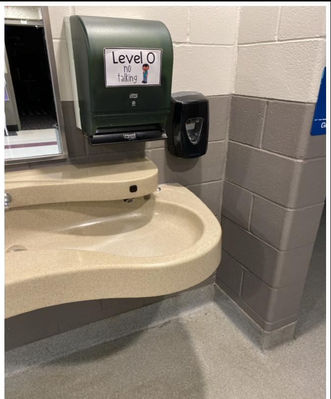
2/8/2024 - 304-38 - Primary School - Across from Room 10 - Right - Out of Order
