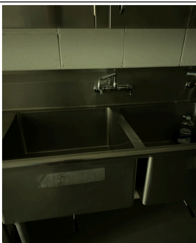
2/7/2024 - 304-58 - Primary School - Kitchen- South Three Bay Sink-Left
