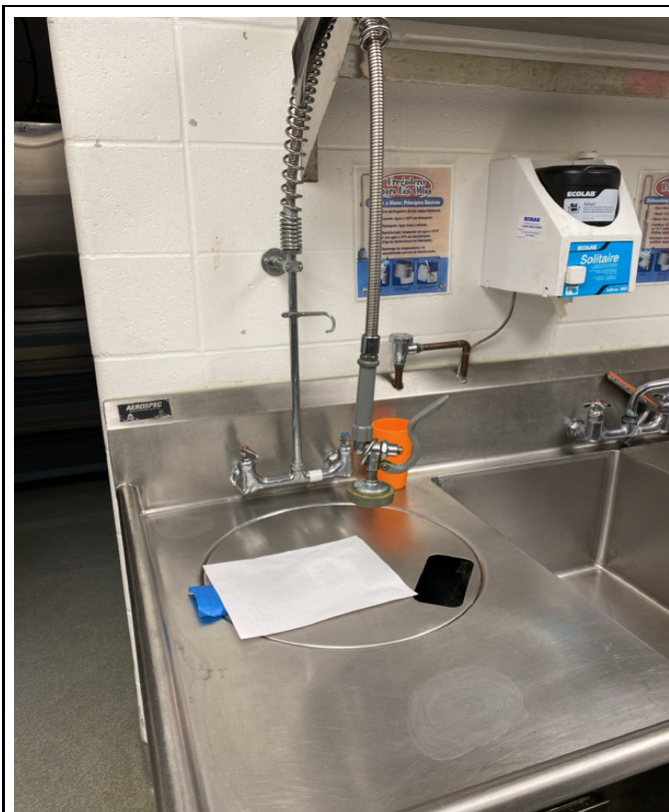
2/8/2024 - 304-53 - Primary School - Kitchen- West Three Bay Sink-Left
