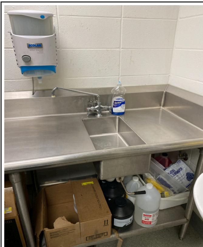
2/7/2024 - 304-57 - Primary School - Kitchen- Northwest Sink
